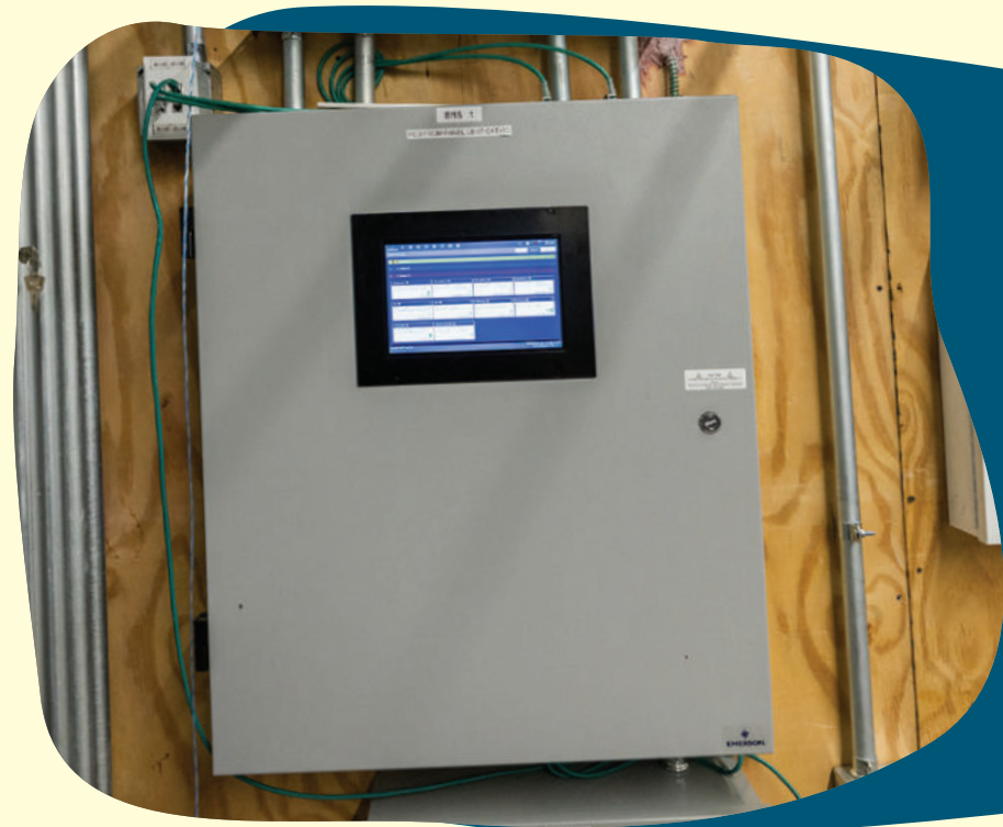
Image Caption: Building Management Systems at Lidl US stores help track and reduce energy consumption.
